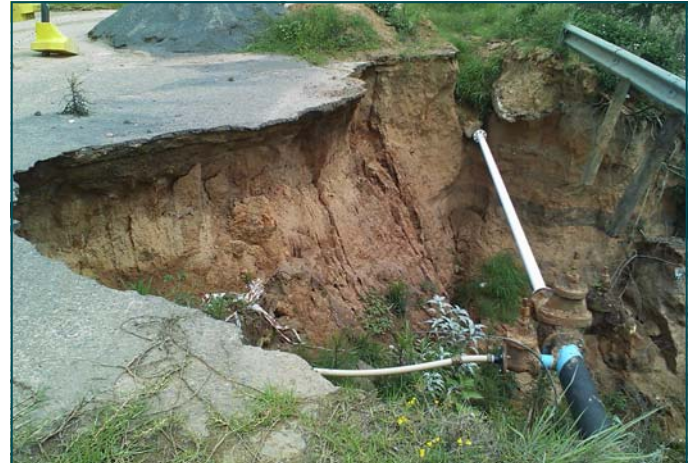
PHOTO 1 - Slip failure showing the pipe failure
