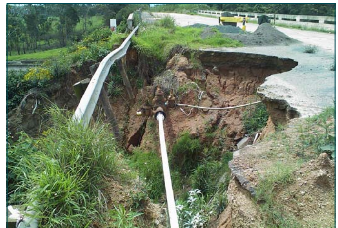
PHOTO 2 - Slip failure showing the impact on the road
