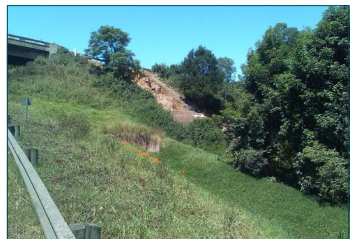
PHOTO 3 - Slip failure as seen from the N3
