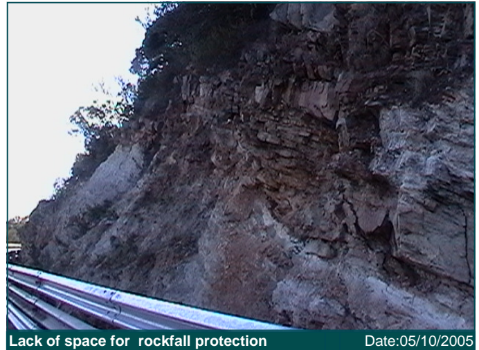
Lack of space for rockfall protection Date:05/10/2005
