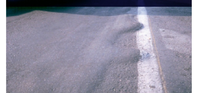
Rutting and shoving
