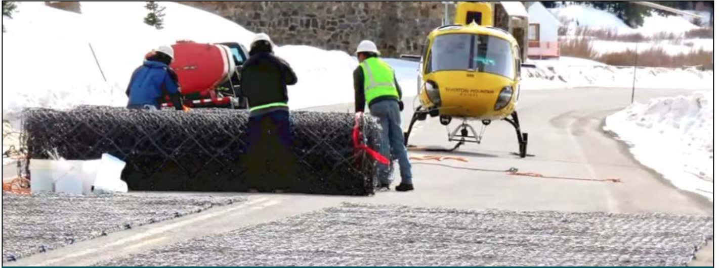
Rolls of HEA Panel are rolled out for loading onto helicopter for installation
