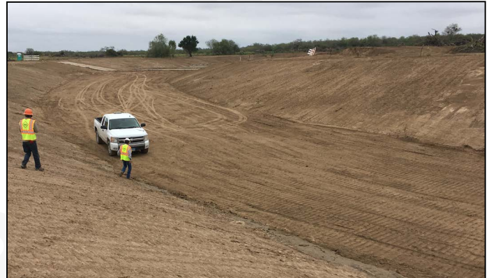
Eroded channel before installation
