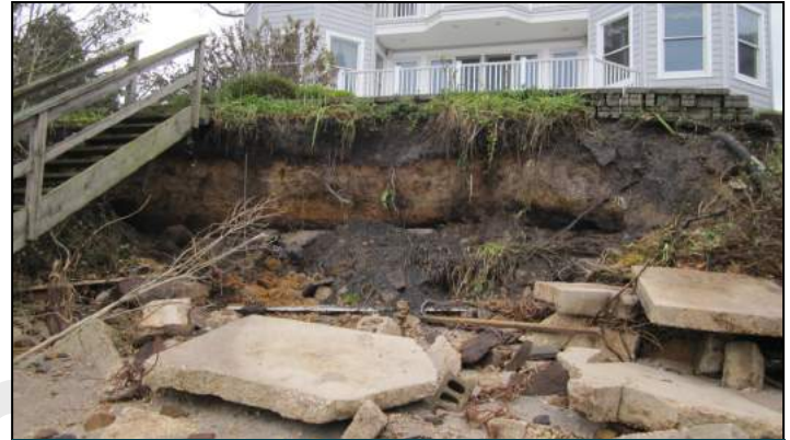
Damage caused by Sandy in October 2012
