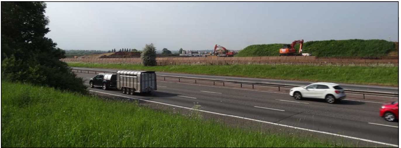
The acoustic barrier had reached 3 m high along its whole length by may 2016
