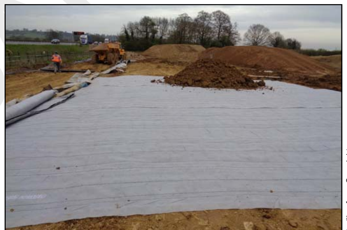
The drainage geocomposite is placed in layers horizontally on the unreinforced area of the acoustic bund
