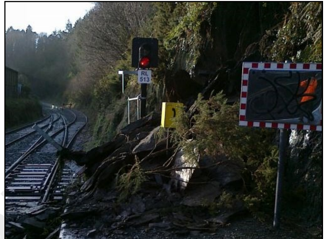
After slope failure
