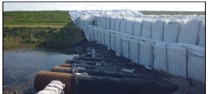
FlexMac units crossing drainage tubes
