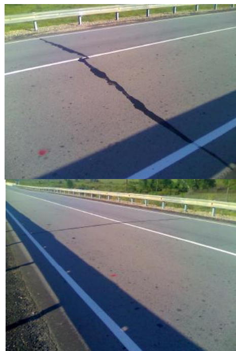
Fig.2 (a) Transverse crack on experimental section ПК 143+39 (b) Transverse crack on experimental section ПК 143+50
