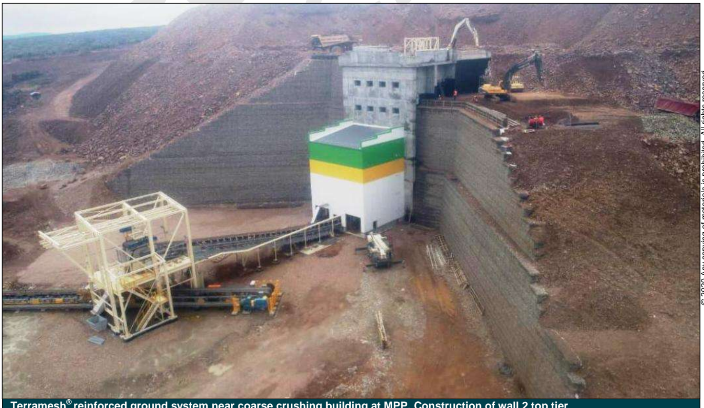
Terramesh® reinforced ground system near coarse crushing building at MPP. Construction of wall 2 top tier
