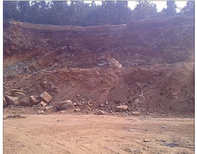
Photo 1: Site - After landslide
