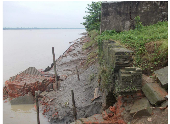
Photo 1 : Existing damaged Compound Wall
