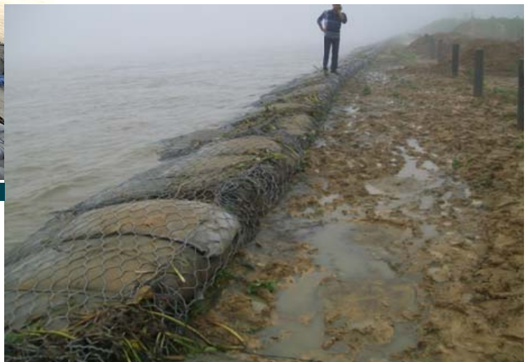
Photo 7 Condition of MacBags™ & River Bank during Flood
