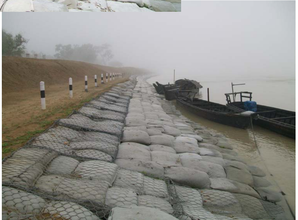
Photo 8 & 9 : Condition of MacBags™ & River Bank after flood
