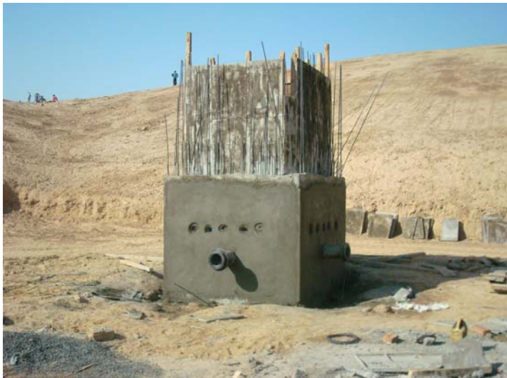
Photo 9,10. Leachate Collection tank
