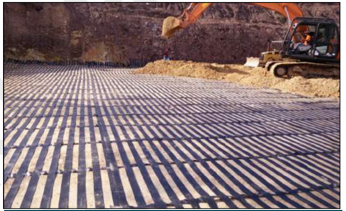
Paralink installation, Nov 2015
