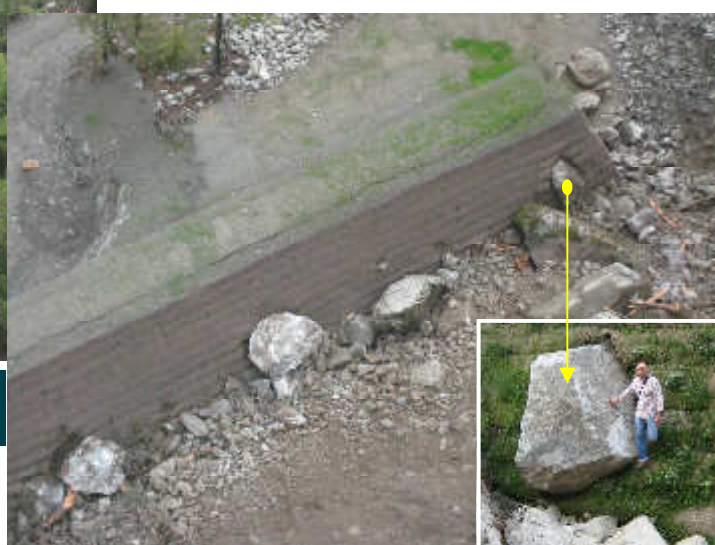
Fig 14. Close-ups of the blocks which struck the upstream embankment
