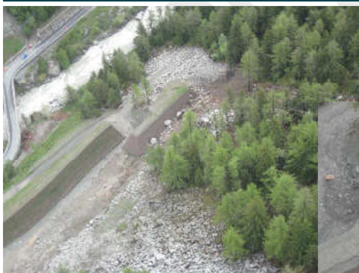
Fig 13. General view of the two embankments in July 2008 after the collapse of a cascade of blocks (>10,000kg)
