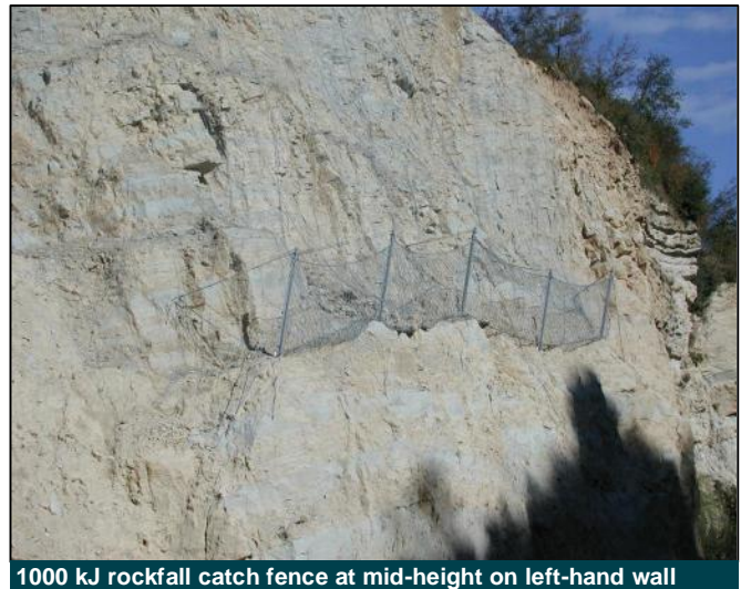
1000 kJ rockfall catch fence at mid-height on left-hand wall
