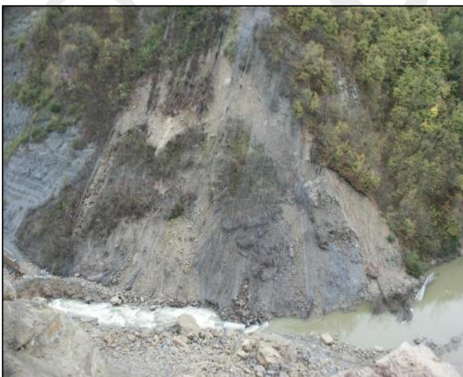
Panoramic view of the road 15 days after the rock fall with the soil landslide before remedial works.
