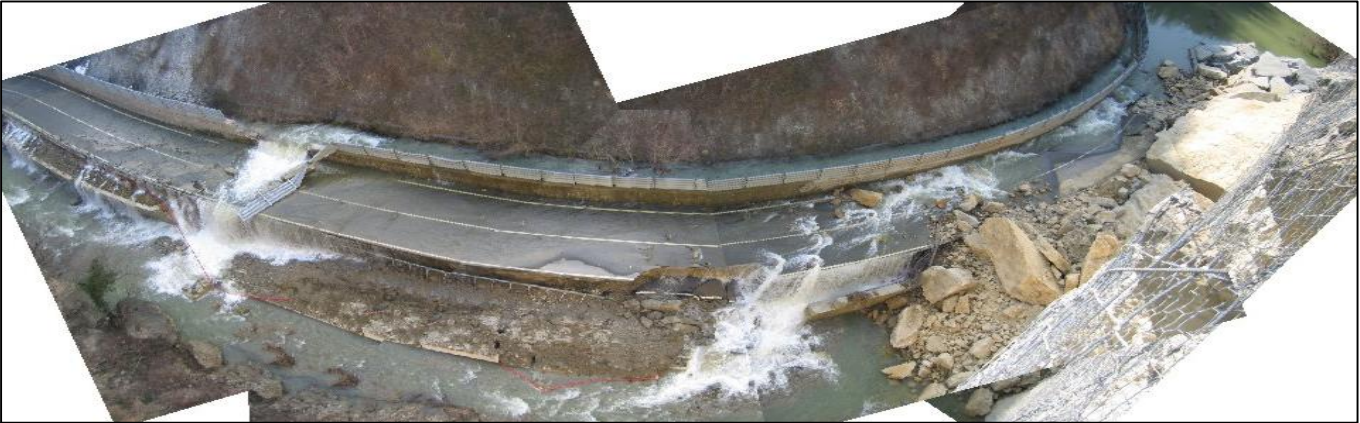
Panoramic view of road just after collapse of rock wall
