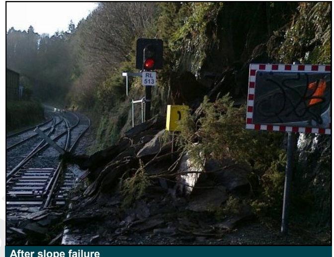
After slope failure
