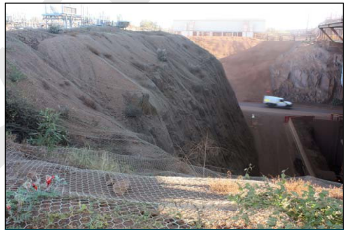
One of the slopes protected with double twist rockfall mesh
