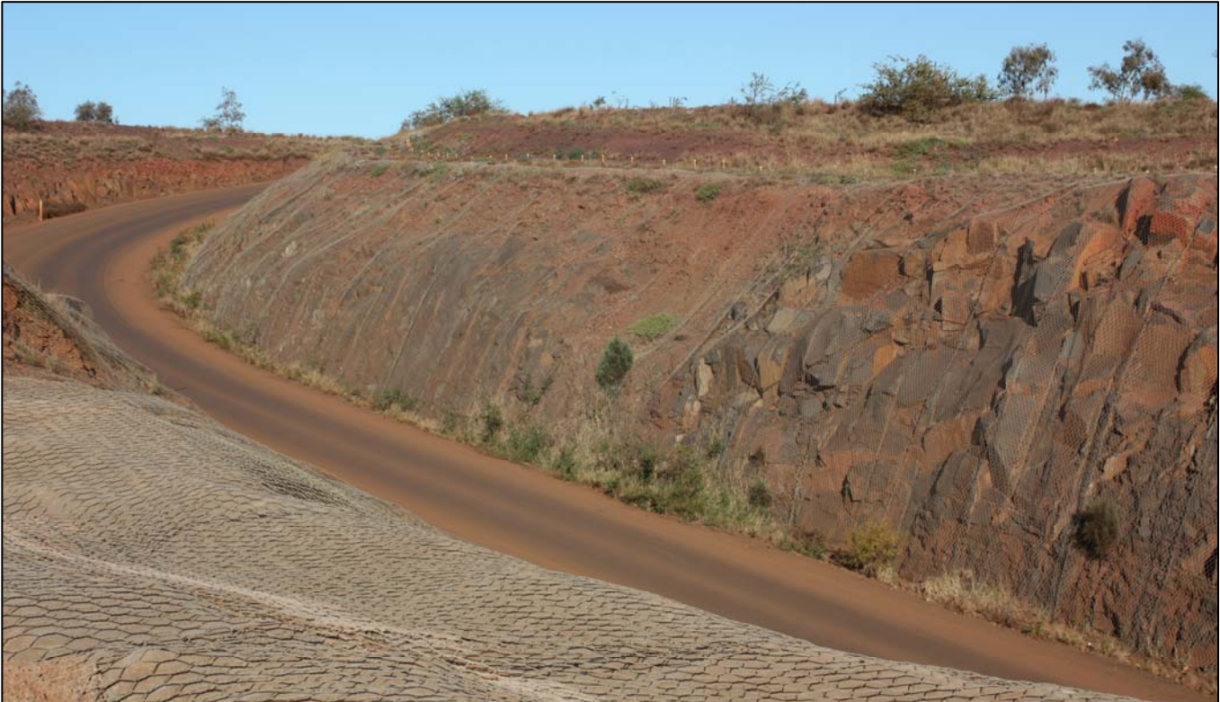
View of the installed double twist mesh on one of the rock slopes
