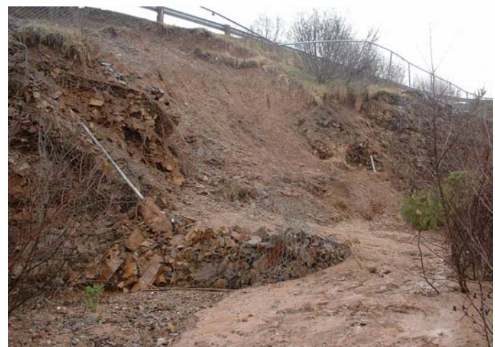
Failed Gabion Retaining Wall, May 2005
