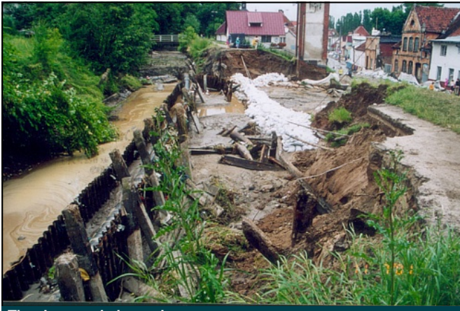
The damaged channel
