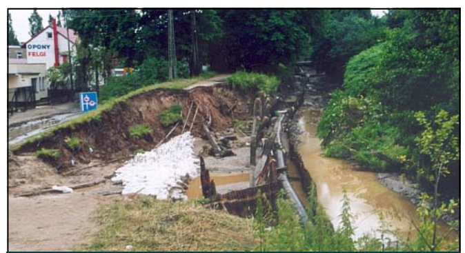
Aftermath of flood
