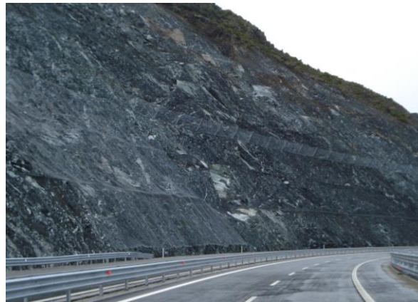
Figure 4. Rockfall protection systems: drapery and catch fences
