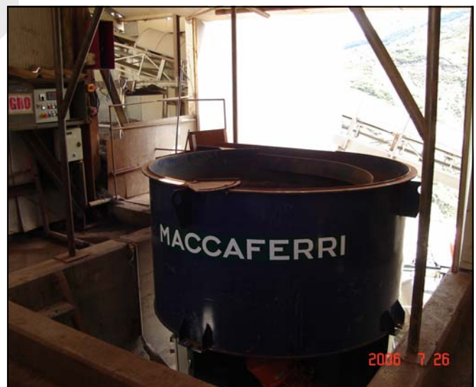
Maccaferri DOSO fibre dosage equipment within concrete plant
